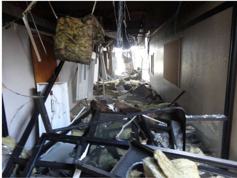
Damage at West Intermediate School
